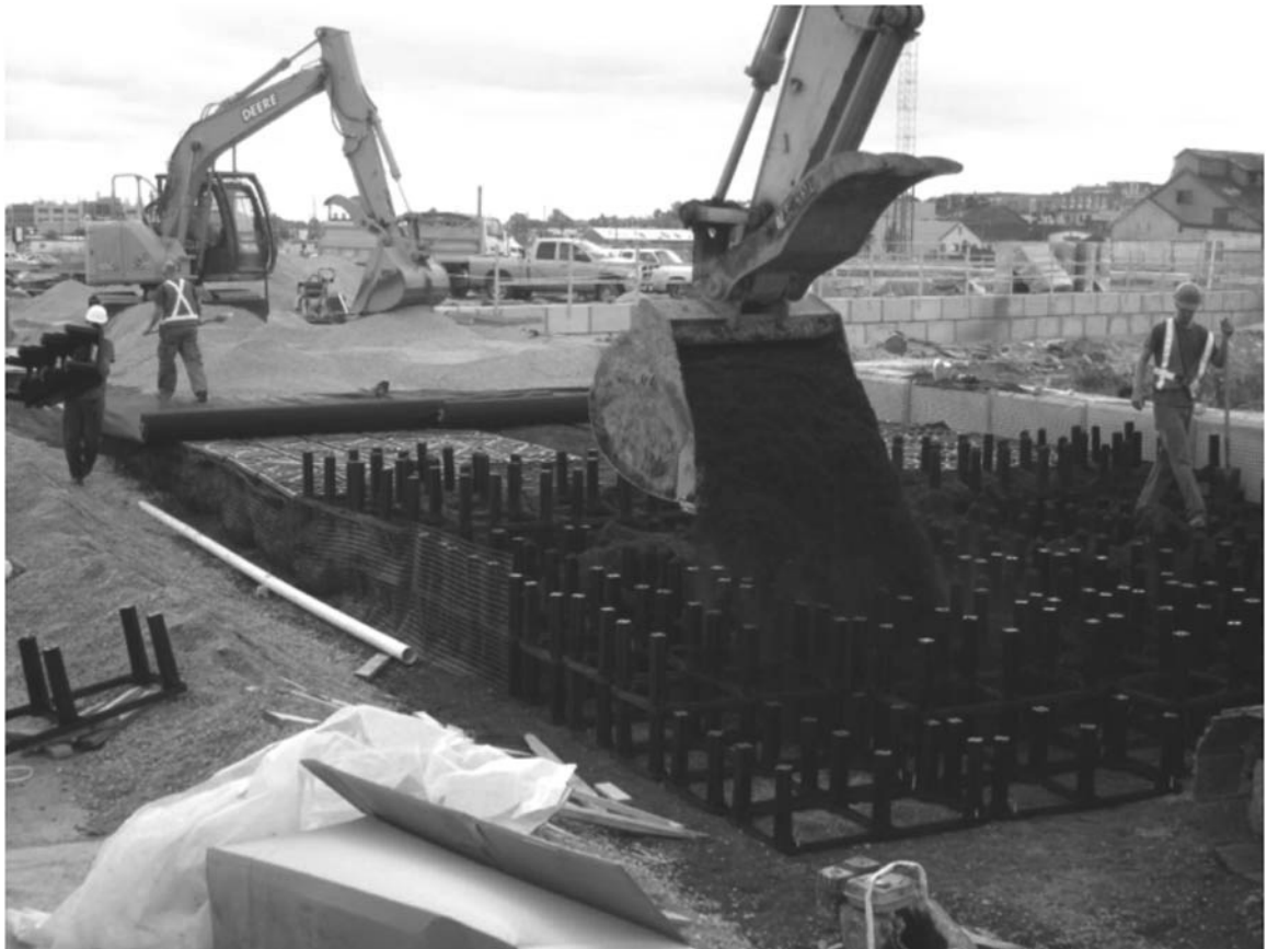
Suspended paving system “Silva Cells” being installed in Vancouver, BC. A wide range of soil types can be used to fill the cell system, which is capable of supporting the weight of large trucks.
